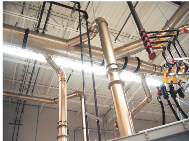
PSP® header and process tool connections installed in new SSP manufacturing facility.
