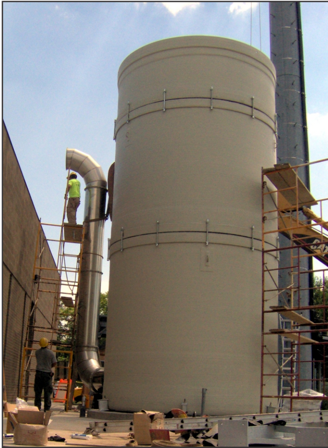
Plumbing PSP® duct and new BioWay multi-stage bioreactor.
