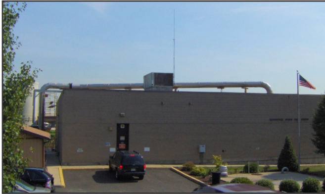
Woodbridge Ave Pump Station with PSP® duct running across roof to bioreactor.
