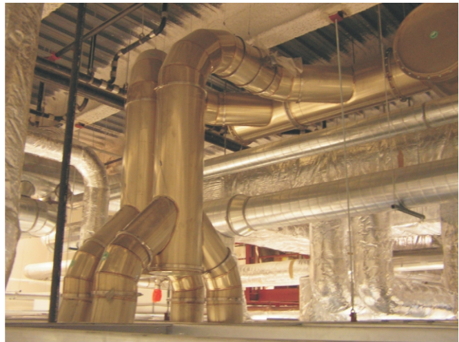
Interstitial level of Weaver Lake 3 facility with PSP® duct shown in the foreground with connection to horizontal header.
