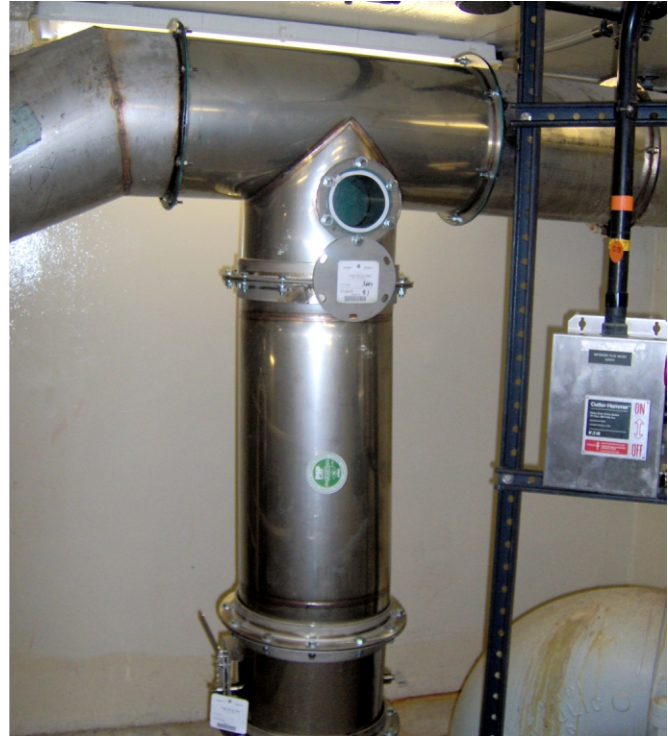
PSP® duct installed at a NYC DEP WPCP.
