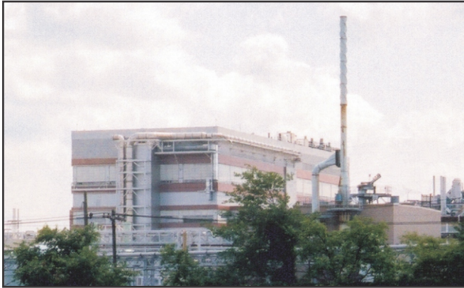
Completed project with PSP® duct installed on building exterior.
