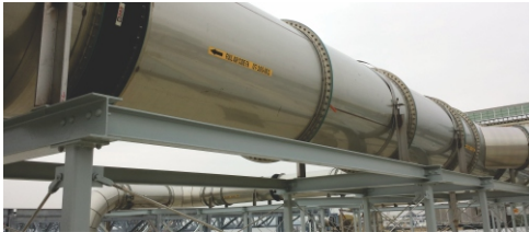
Dewatering facility odor control duct.
